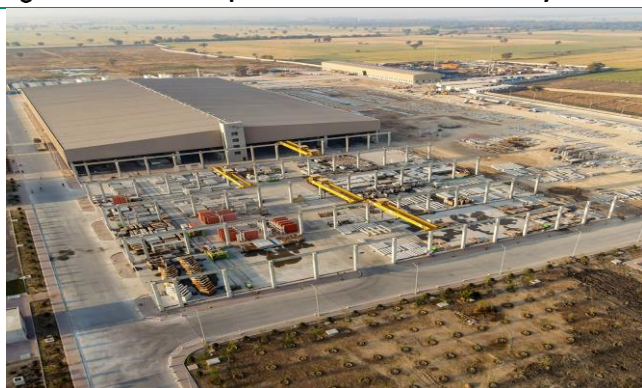
Fig 11: Precast - Comprehensive view of the facility
